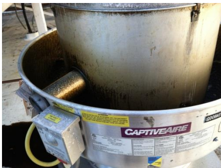
Dysfunctional filters result in grease on roof
