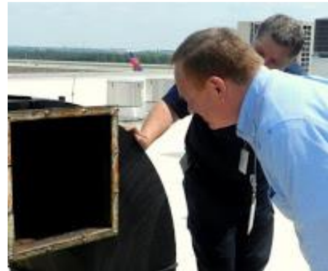
Typical exhaust duct emptying airborne grease
